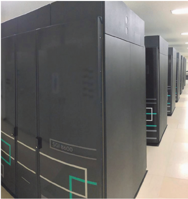
Fig. 1. Photo of the supercomputer (HPE SG18600) in this study.
